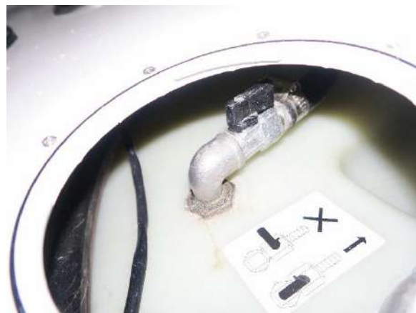
Fuel shut-off valve
