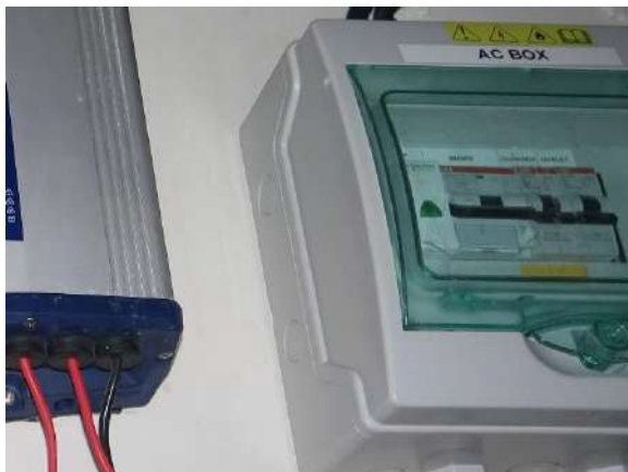
Residual current and main circuit breakers
