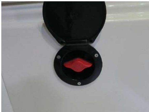
Windlass and bow thruster circuit breaker
