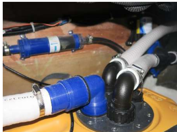
Black water tank
