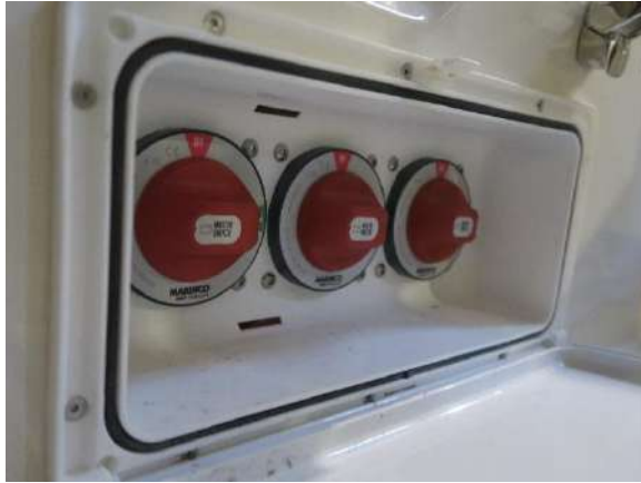
Main circuit breakers
